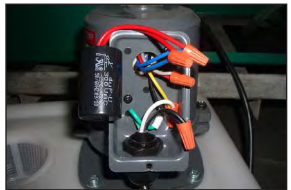
Figure 50. Pump motor wiring and capacitor (M2).
