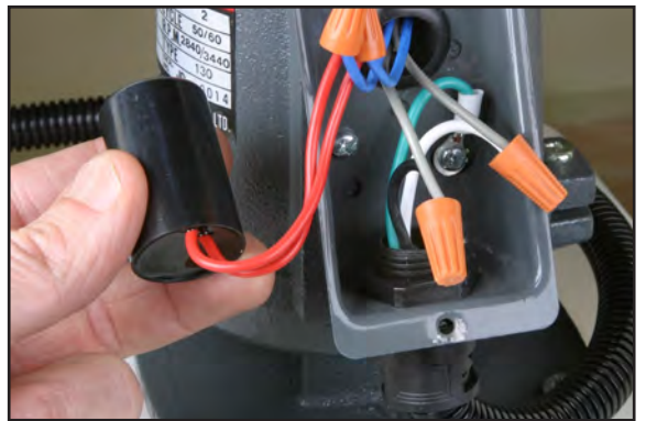
Figure 50. Pump motor wiring and capacitor (M2).
