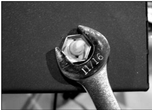
Figure 8.18 Install the speed control (rheostat). The speed control mounts to the decorative cover removed in Step 5. Insert the stem of the speed control through the hole located on the right side of the cover. Secure with the pal nut using an 11/16 in. (17.5 mm) wrench. Attach the black and white wires routed under the appliance indicated in Figure 8.13 , on page 34, to the two speed control wires. Push the speed control knob onto the stem and re-attach the decorative cover. Secure the wires up and out of the way using the zip tie provided.
