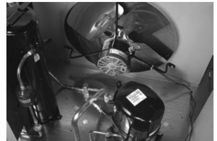
Typical Outdoor Unit with throwaway liquid-line filter and sight glass
