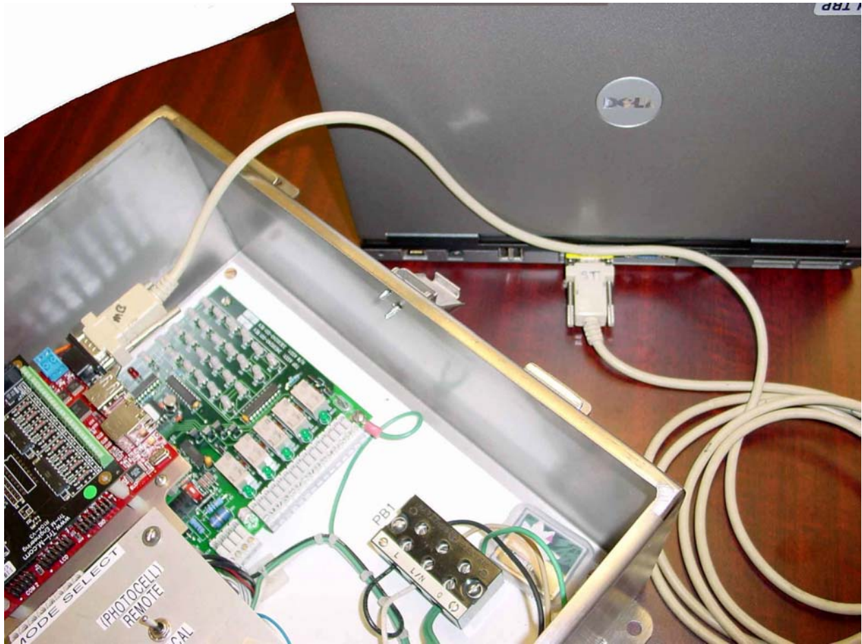
Figure 3.7-1 PC to PLCHMR RS-232 Serial Port Interface Cable Connections
