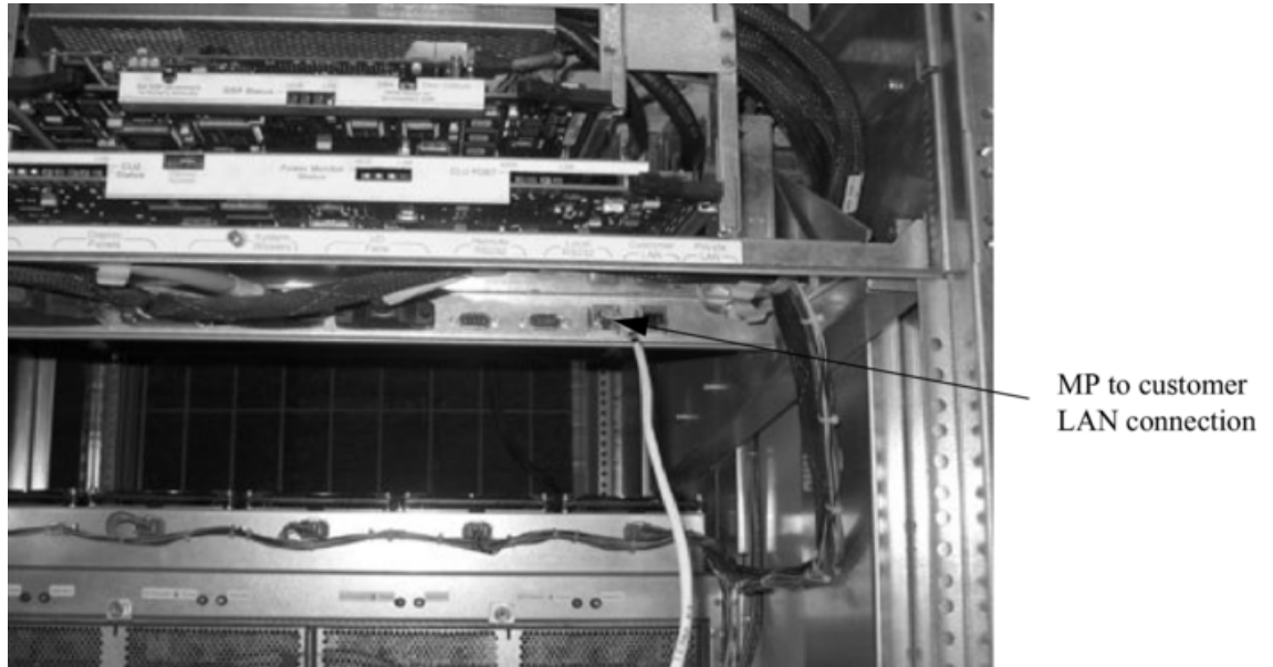
Figure 3-38 MP LAN Connection Location
